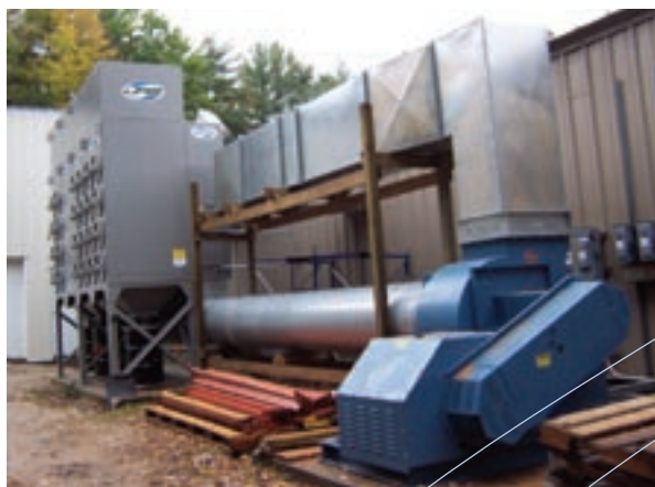
A SFC 48-4 with an air distribution module and ground mount blower collects plastic dust.
